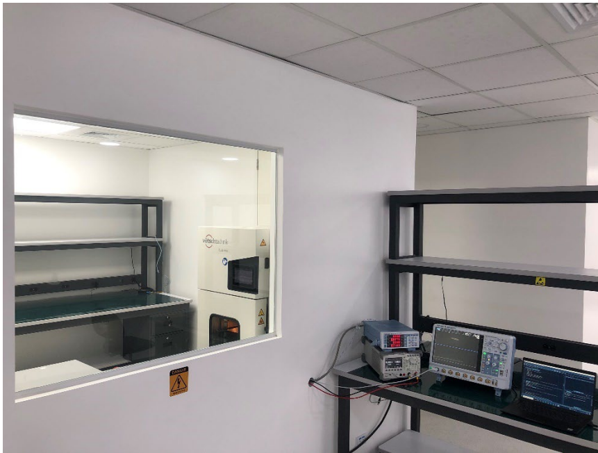
Figure 11 – High Voltage Test Set-up.
